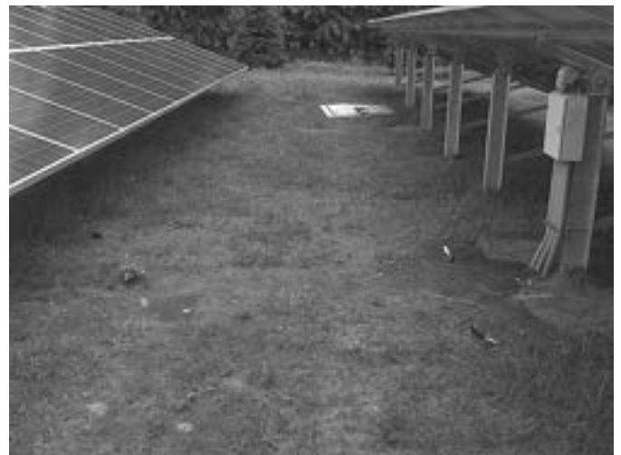
Fig. 5. Site showing the initiation of bare ground below the panels, which increases the potential for erosion (photo by John Showler, reprinted with permission)
